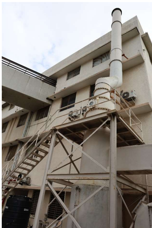
Wet Scrubber to Control Air Pollution
