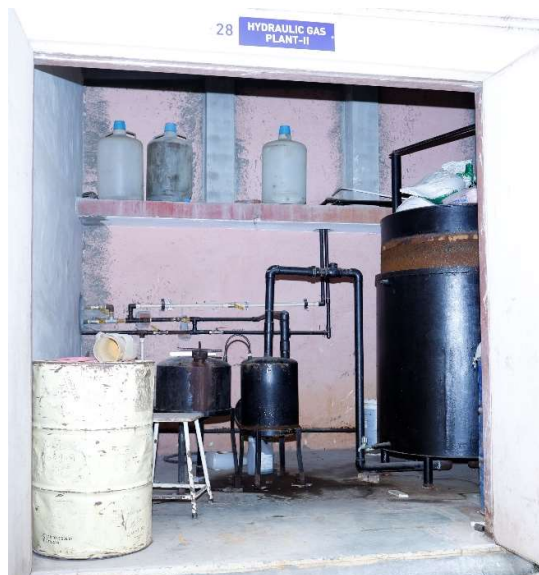
Hydraulic Gas Plant
