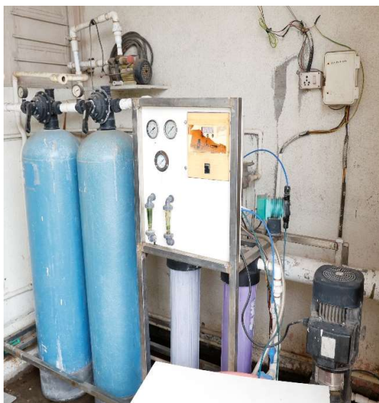
Water Softener System
