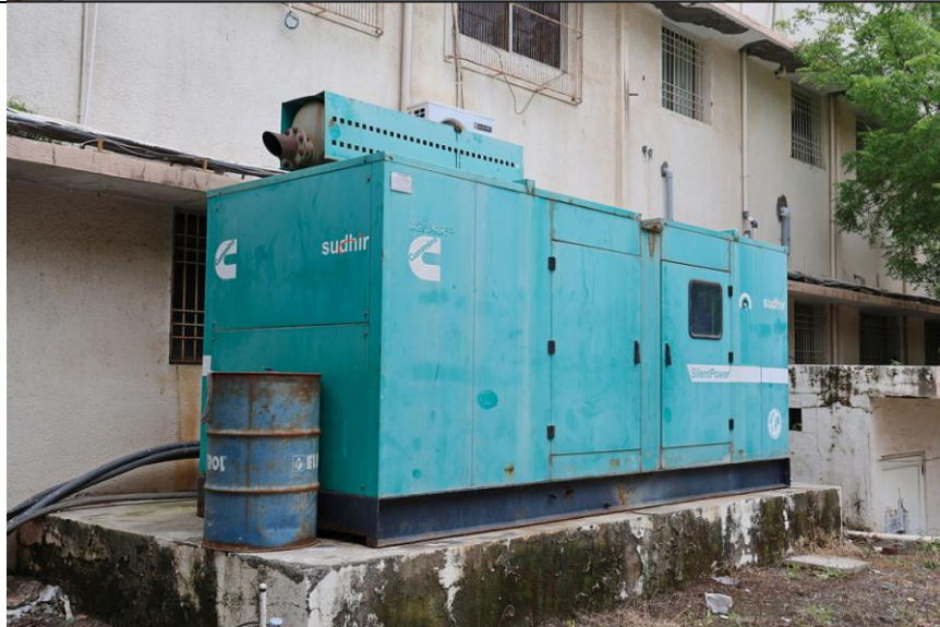
Eco-friendly Power Backup Generator
