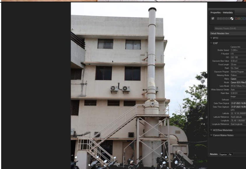
Air Pollution Control Measures - Alkali Wet Scrubber for removing Acidic fumes generated in Chemical Sciences Laboratories
