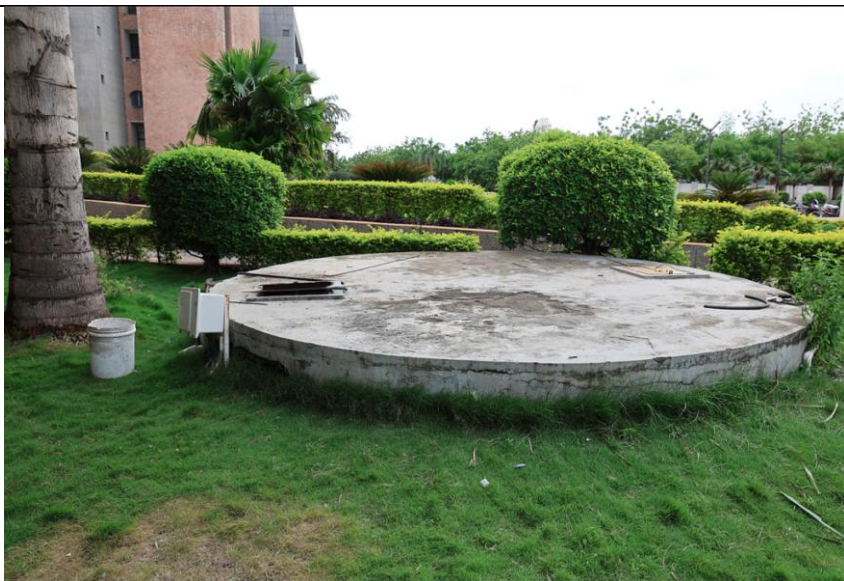
Rain Water Harvesting System
